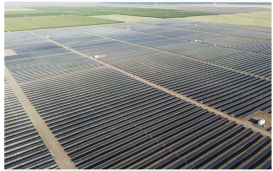
The 73 MW Luciana Solar Project in Ducor, CA. (Courtesy: Idemitsu Renewables)
